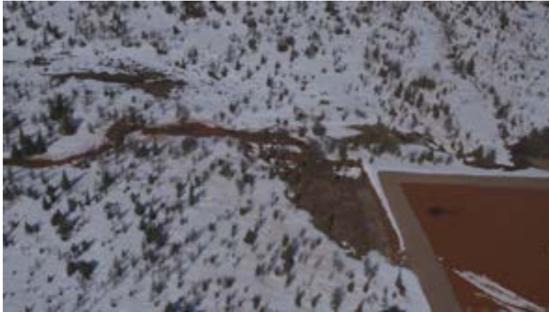
Figure 3. At the culvert outlet, water had overtopped the snow-filled outlet ditch, spreading into the adjacent wetland rather than being channelled into Goodream Creek.
