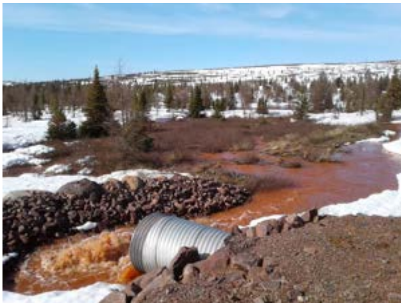
Figure 4. Water flowing from culvert into adjacent wetland.
