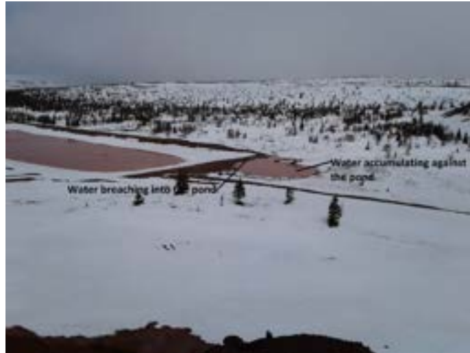
Figure 1. Breach opening at the SE corner of SP3 allowed runoff to enter and pool against and berm.
