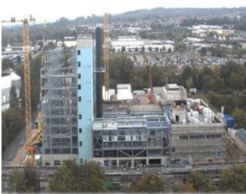
Boehringer Ingelheim, Germany, 36 – 68 t/h Biomass, Waste Wood, Sorted Waste – RDF
