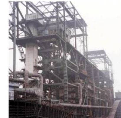
Jinan Iron & Steel Group, China, 39 t/h Waste Gas Quantity, 115.000 Nm 3 /h
