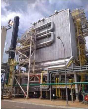
BASF, Malaysia, 2 x 100 MWth, 17 Mwel Natural Gas
