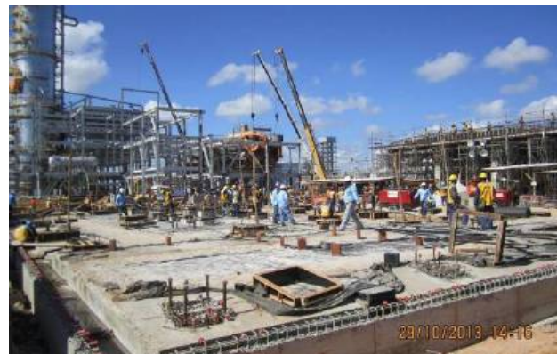
BASF, Brazil, 98 t/h Liquid and Gaseous Residues
