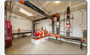
Sprinkler Riser Room
