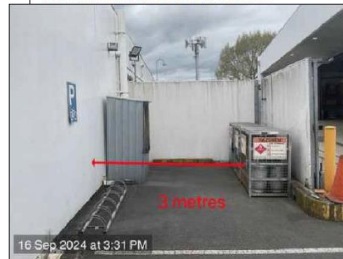
PICTURE 4 : ZONE 2 180KG LPG CYLINDER STORAGE CAGE AS SHOWING 3 METERS TO THE MAIN BUILDING EXTERIOR WALL
