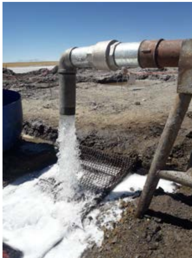
Figure 7.56 Pumping Well W18-05
