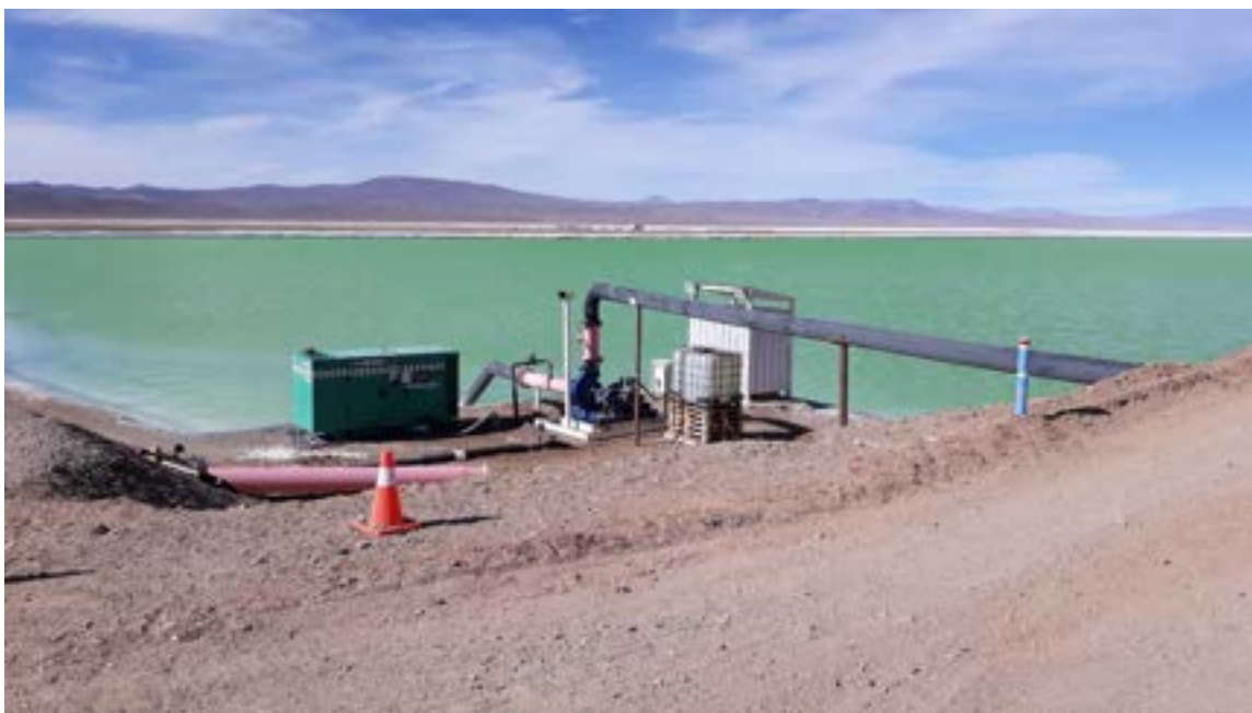
Figure 14.6 Evaporation Ponds – Transfer Pump Station
