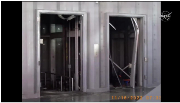
Figure 4. ML-1 elevator damage: elevator doors on ML-1 after the Artemis I launch. Source: NASA.
