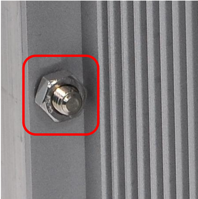
Ground screw of the switch
