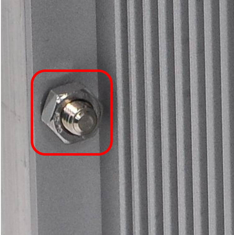
Ground screw of the switch
