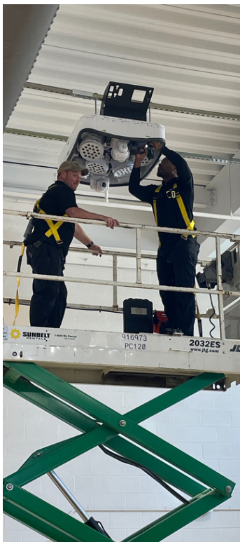
Dorothy Technology Installs new Lü System
