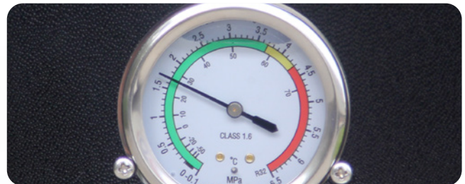
Refrigerant System Pressure Gauge
