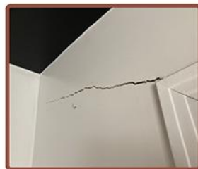
Drywall cracks are common signs of foundation problems.
