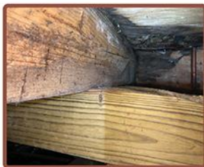
Moisture related wood rot can be a cause of sagging floors.
