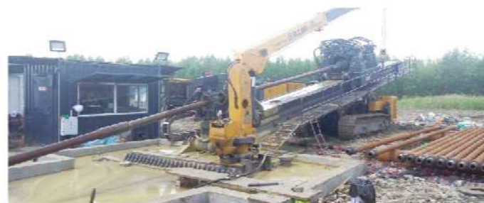
XZ6600, Water supply pipeline, \Phi 813\text{mm} , 3000m
