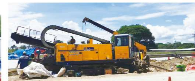
XZ1350, Thailand, Telecom pipeline
