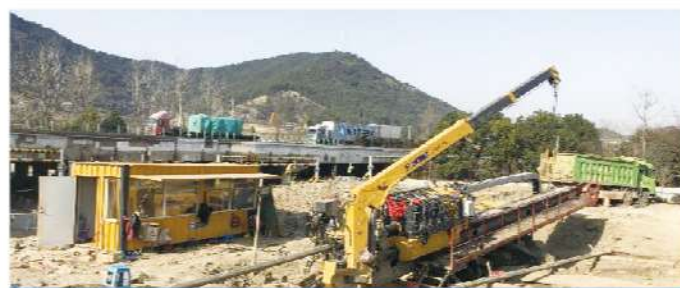
XZ5060, Oil pipeline, \Phi 1016\text{mm} , 1300m
