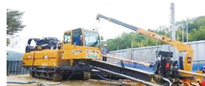
XZ3600, Korea, Water supply pipeline
