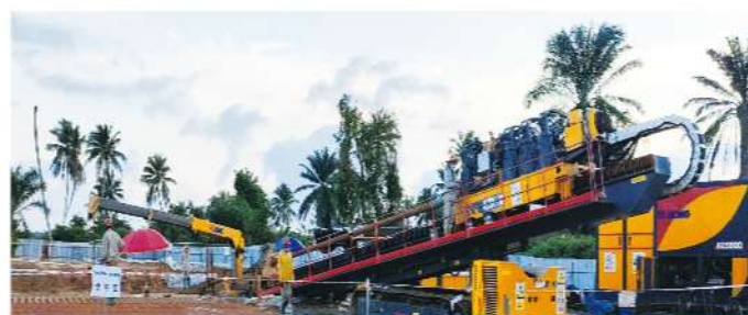
XZ6600, Niger and Benin, Oil pipeline
