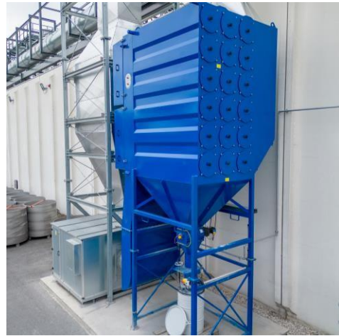
Figure 9: The installed, low-maintenance filter system
