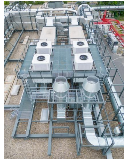
Figure 5: Adiabatic cooling units from a bird's eye view
