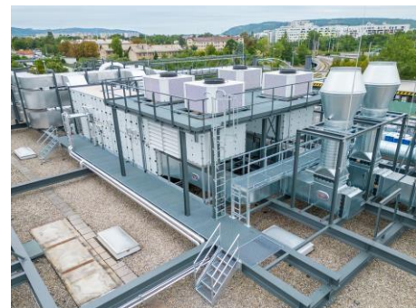
Figure 4: The new adiabatic cooling system on the roof of Kansai Helios
