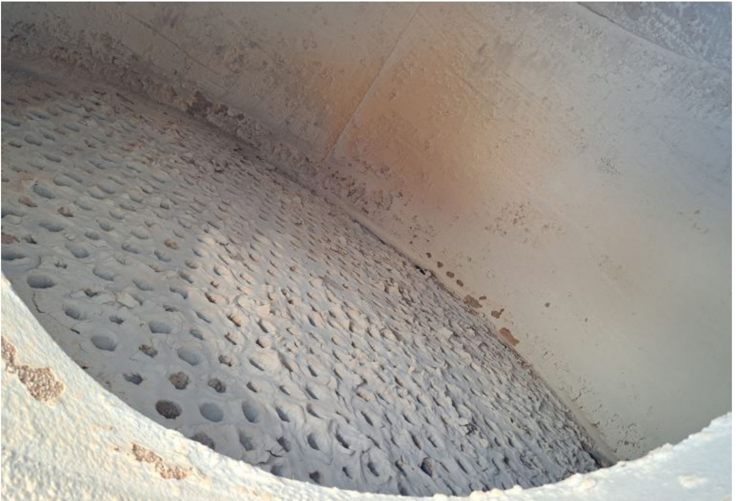
Image 02: The contaminated heat exchanger: Over the years, deposits have formed that affect efficiency and performance. A comprehensive overhaul is necessary to optimize heat recovery.
