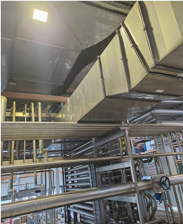
Image 02: Piping in stainless steel and with special suspension systems for the textile air hoses
