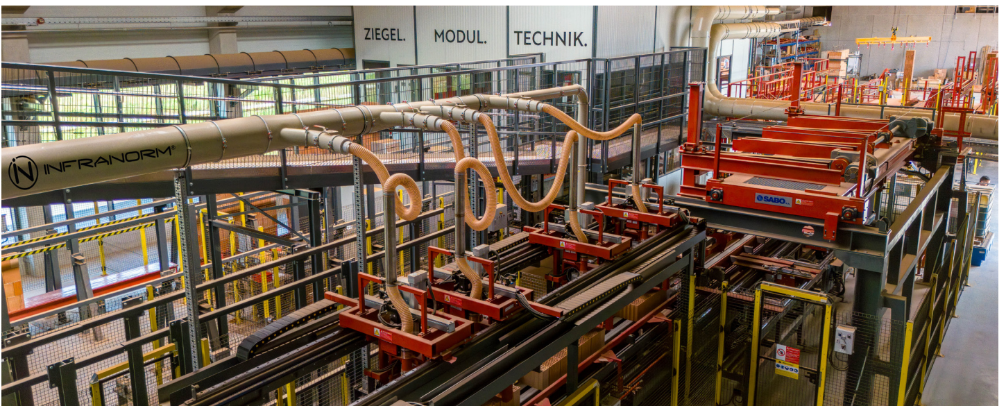
Picture 05: With an extraction capacity of up to 42,500 m 3 /h and 4800 Pa negative pressure, the system ensures optimum dust collection – even in 100 % recirculation mode.
