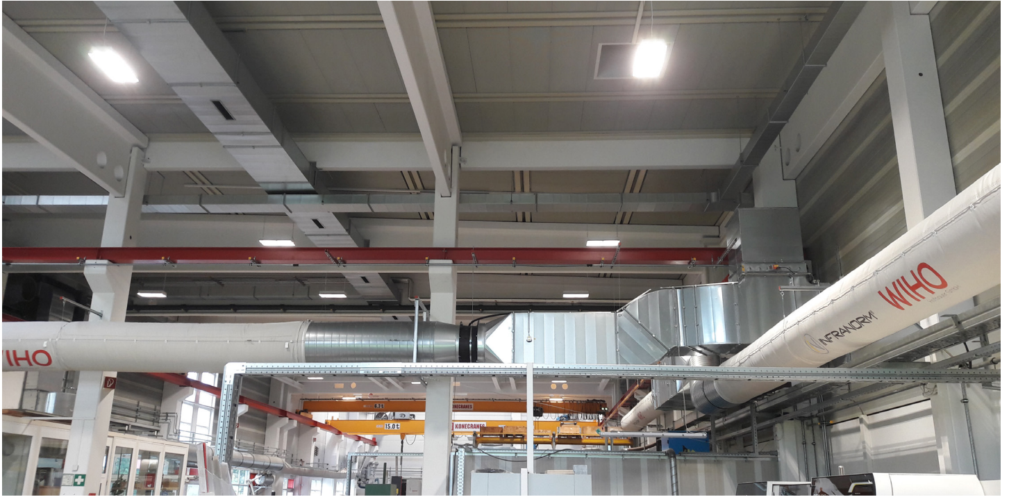
Image 02: Integration of the warehouse cooling system into the existing infrastructure, including air distribution and central system connectivity
