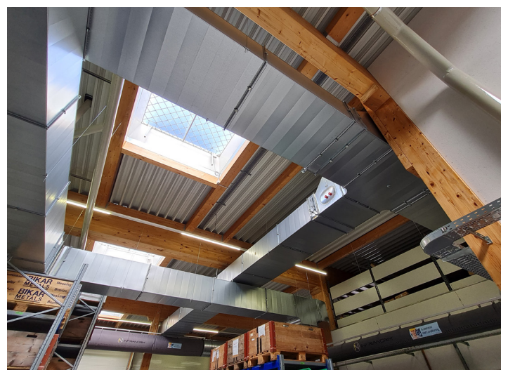
Image 05: Air distribution system for draft-free distribution of conditioned air in the work area
