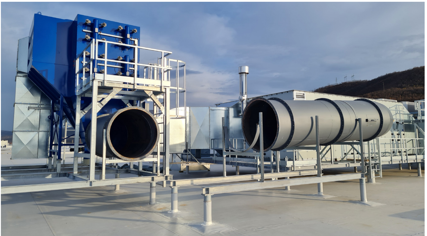
Image 05: Cartridge filter system and air ducting system for capturing welding and grinding fumes in the production hall
