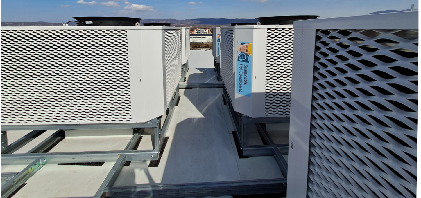
Image 04: Roof-mounted SHC system for energy-efficient industrial building cooling using two-stage adiabatic cooling
