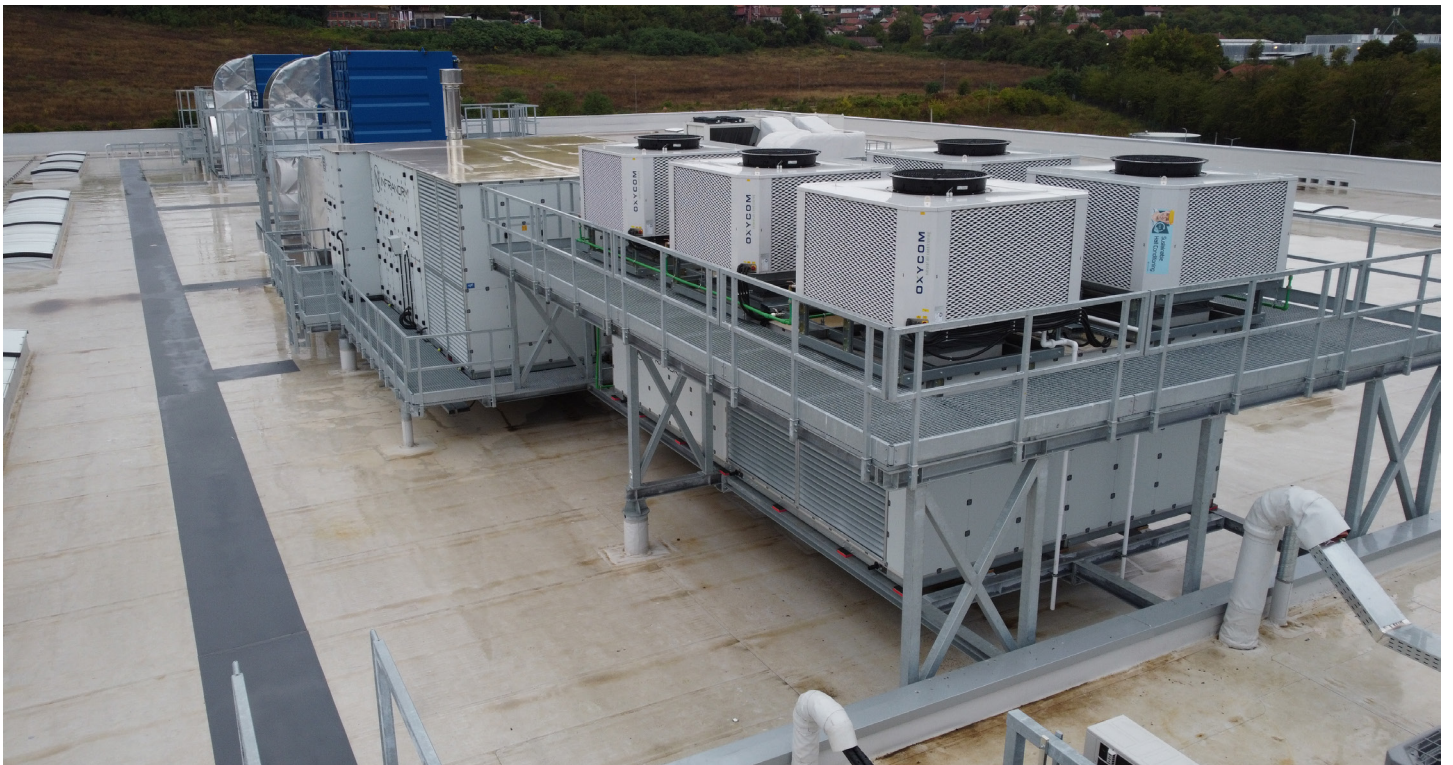
Image 07: Roof-mounted recoolers and SHC components for energy-efficient industrial building cooling
