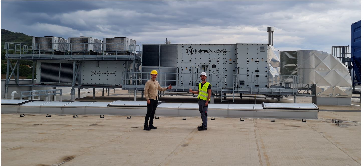
Image 06: Roof-mounted SHC system for energy-efficient climate control of the welding shop
