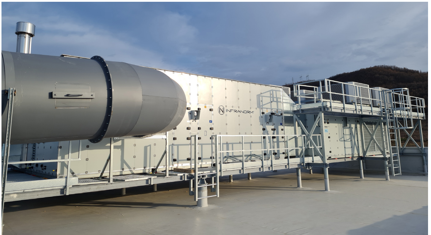
Image 02: Outdoor ventilation and industrial air conditioning system with integrated heat recovery and air distribution for welding operations
