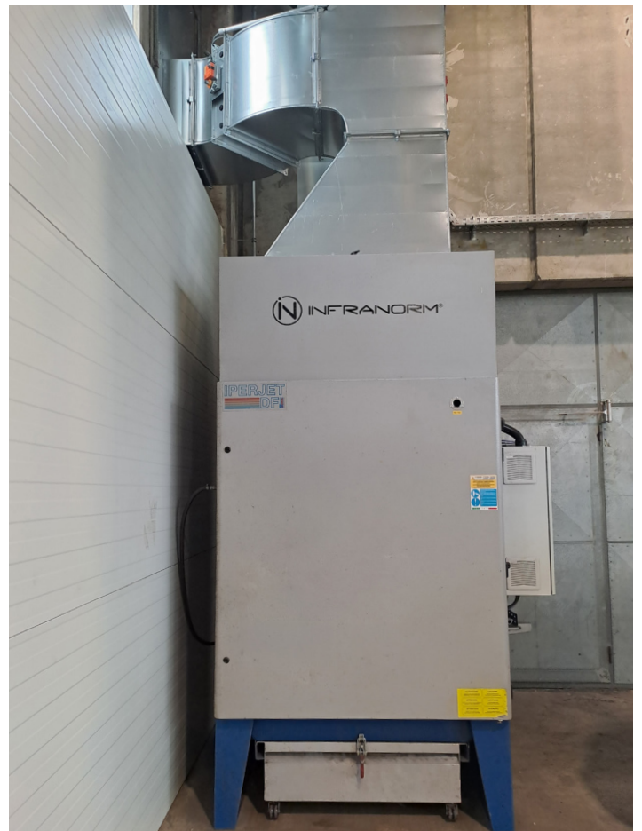
Image 05: Existing filtration system that was integrated into the new overall system as part of the retrofit
