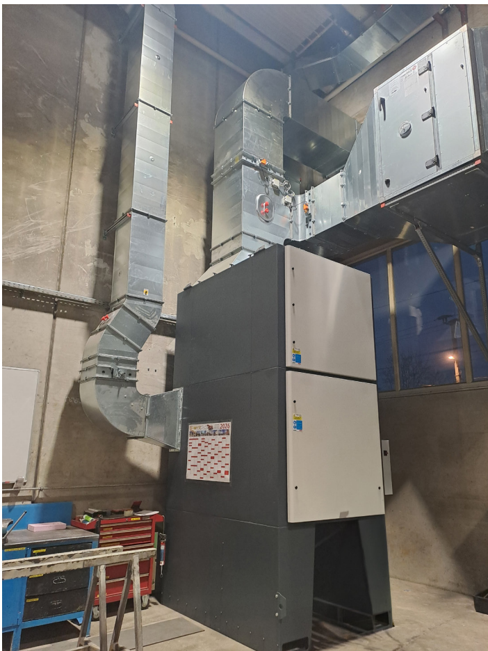
Image 04: New filtration system with integrated ductwork for summer and winter operation
