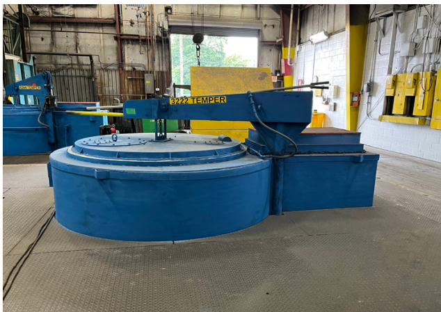
Fig. 1 Typical Pit Furnace
