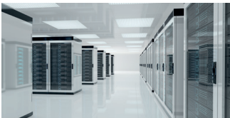
AI Data Servers, Supercomputing
