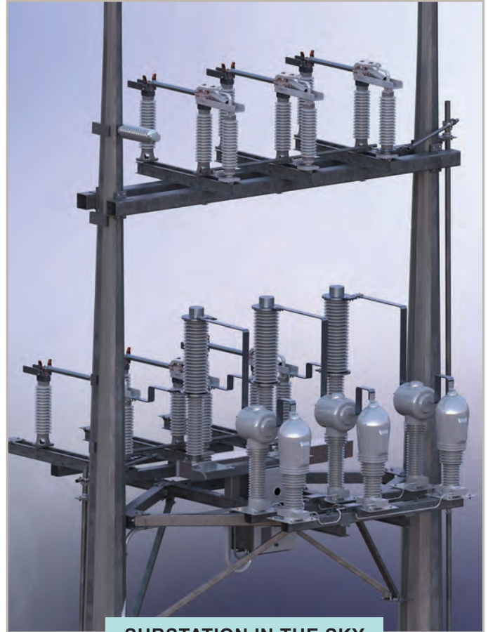
SUBSTATION IN THE SKY
