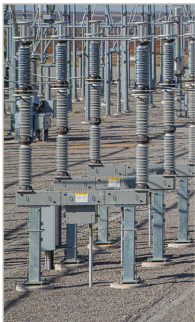
362 kV pictured above
