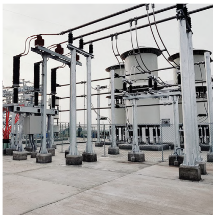
Steel (EAF) 75 MVAR SVC
