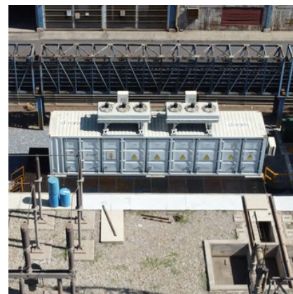
Rolling mill 15 MVAR STATCOM
