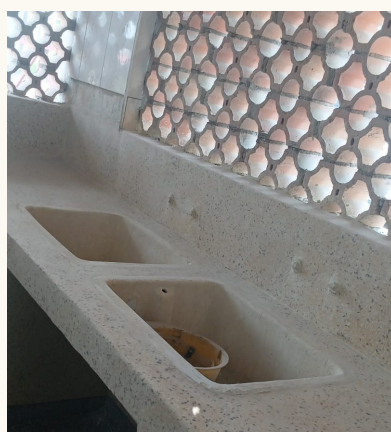
Providence Medical Center Terrazzo sinks & countertops
