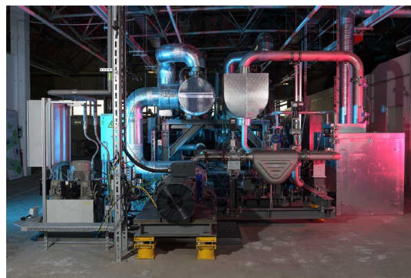
High-temperature heat pump technology in an industrial setting. Source/Copyright: DLR
