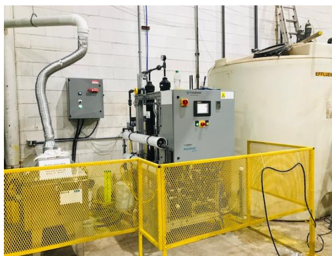
Installation in Montreal (Canada). Capacity : 7,000 L/day
