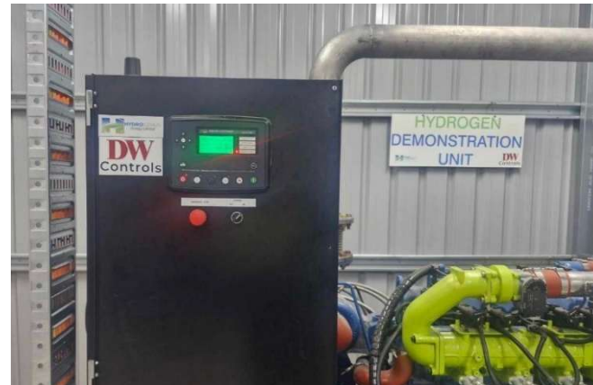
Control Unit for the Ballarat demonstration
