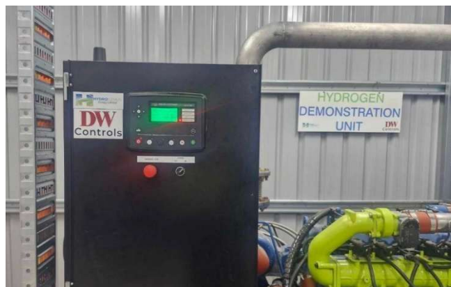
Control Unit for the Ballarat demonstration
