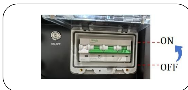
Figure 29 Open the Circuit Breaker on BDU
