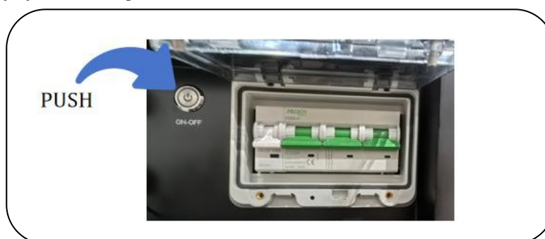
Figure 32 The Power Switch Of Battery Systems
