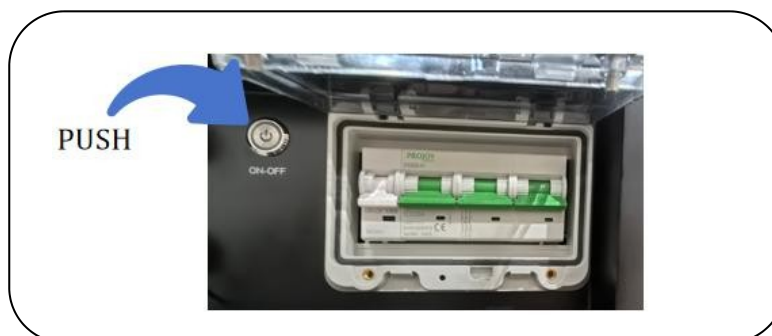
Figure 32 The Power Switch Of Battery Systems
