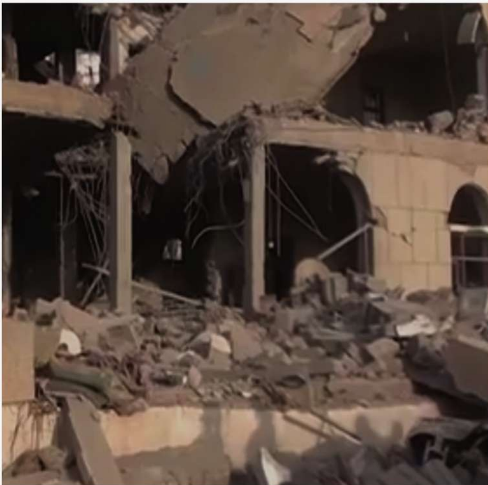
Government Compound in Al-Hazm District, Al-Jawf Governorate, following US airstrikes under "Operation Rough Rider" on March 17, 2025.
