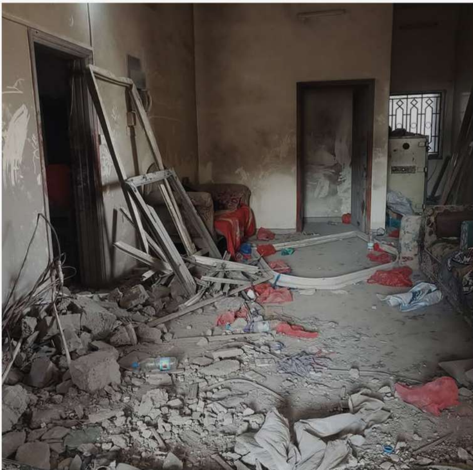
An image from inside the Al-Maswari house showing the destruction of a residential building in Al-Hudaydah Governorate following US
