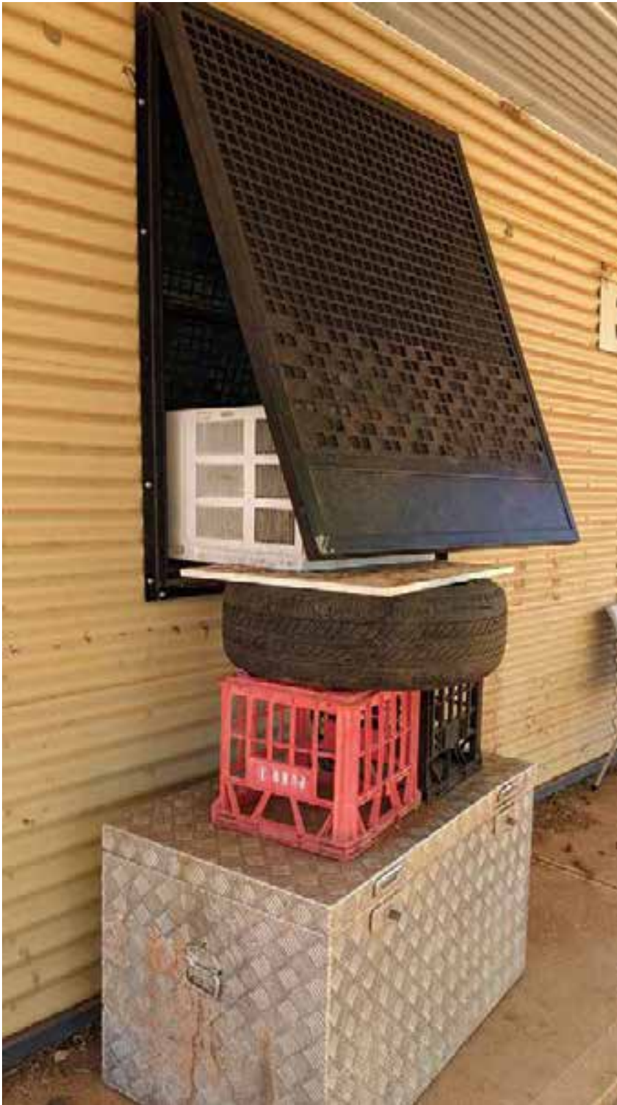
A precariously installed refrigerated air conditioner, below a security screen. Photo: Liam Grealy, 2021.
