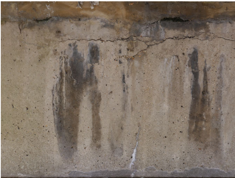
Concrete as microbiome. The darker patches contain cyanobacteria. Bedford Way, London. Photo: Matthew Gandy, 2021.
