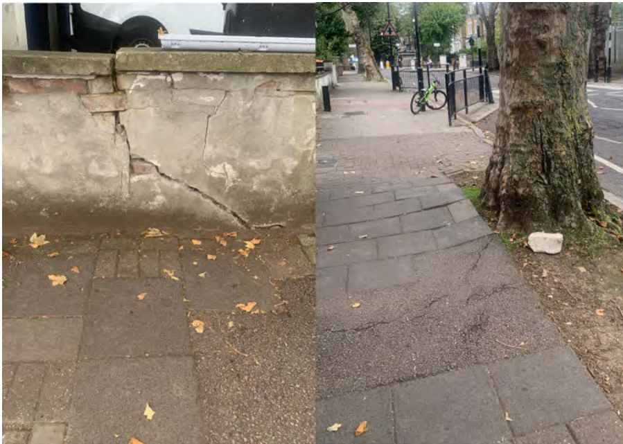
The roots of a London plane tree crack an adjacent wall (left) after meandering below the paved sidewalk (right).
