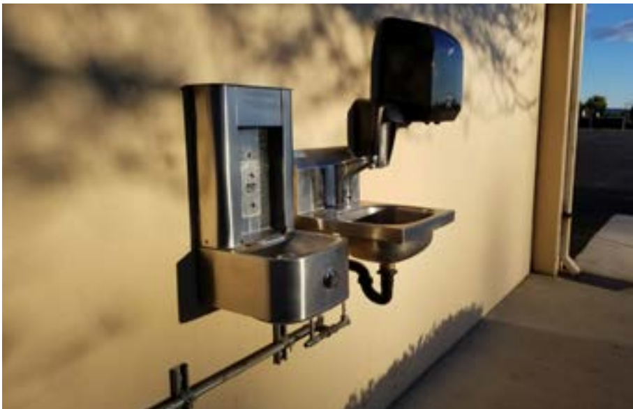
A newly installed filtered water bottle filling and handwashing station at Azusa High School. Photo: Fred Ariel Hernandez, 2023.
