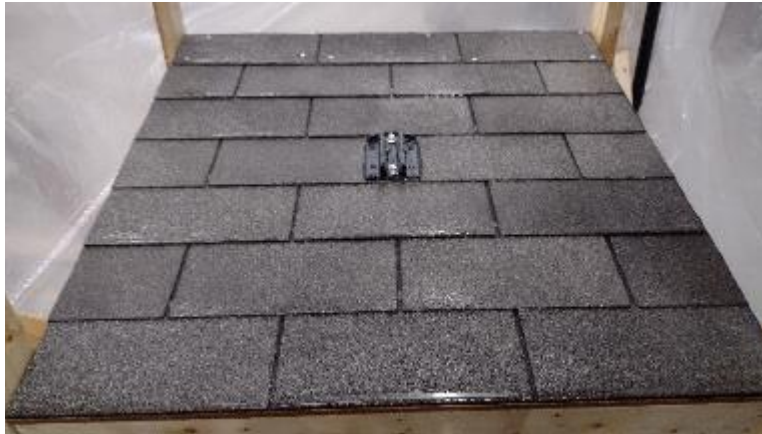
Photo No. 1 SunStack (SSB1) Solar Mount, Top View
