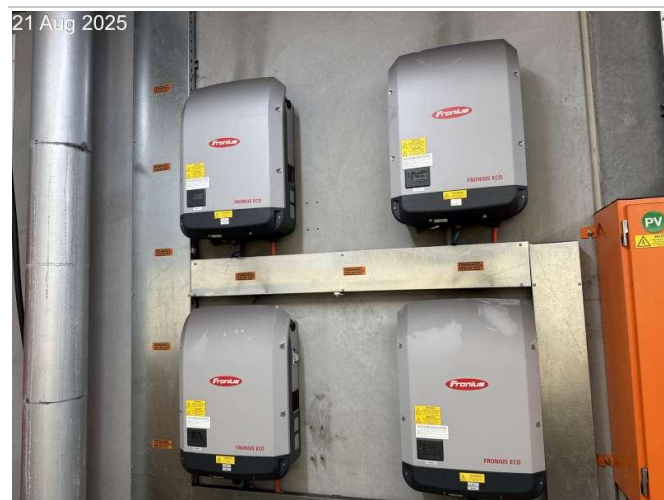
Solar AC System
