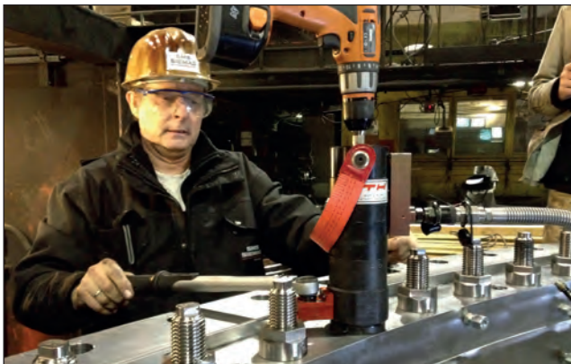
Ladle turret bolt connection.
