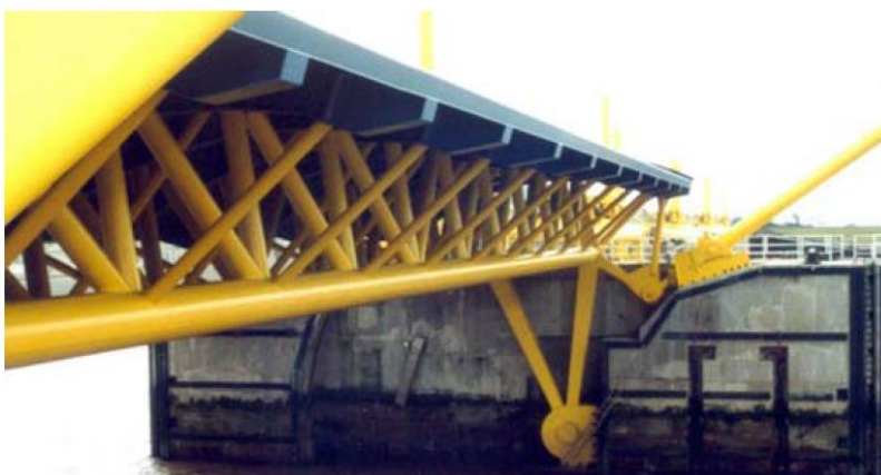
Segment gate of the inland navigation opening in upper position
