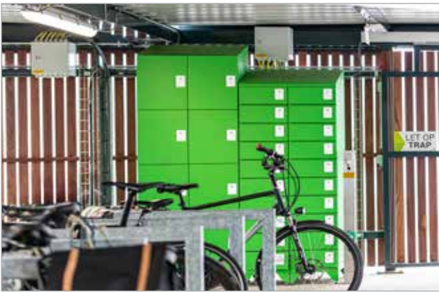
VPK Oudegem - boxes for powering electric bike batteries
