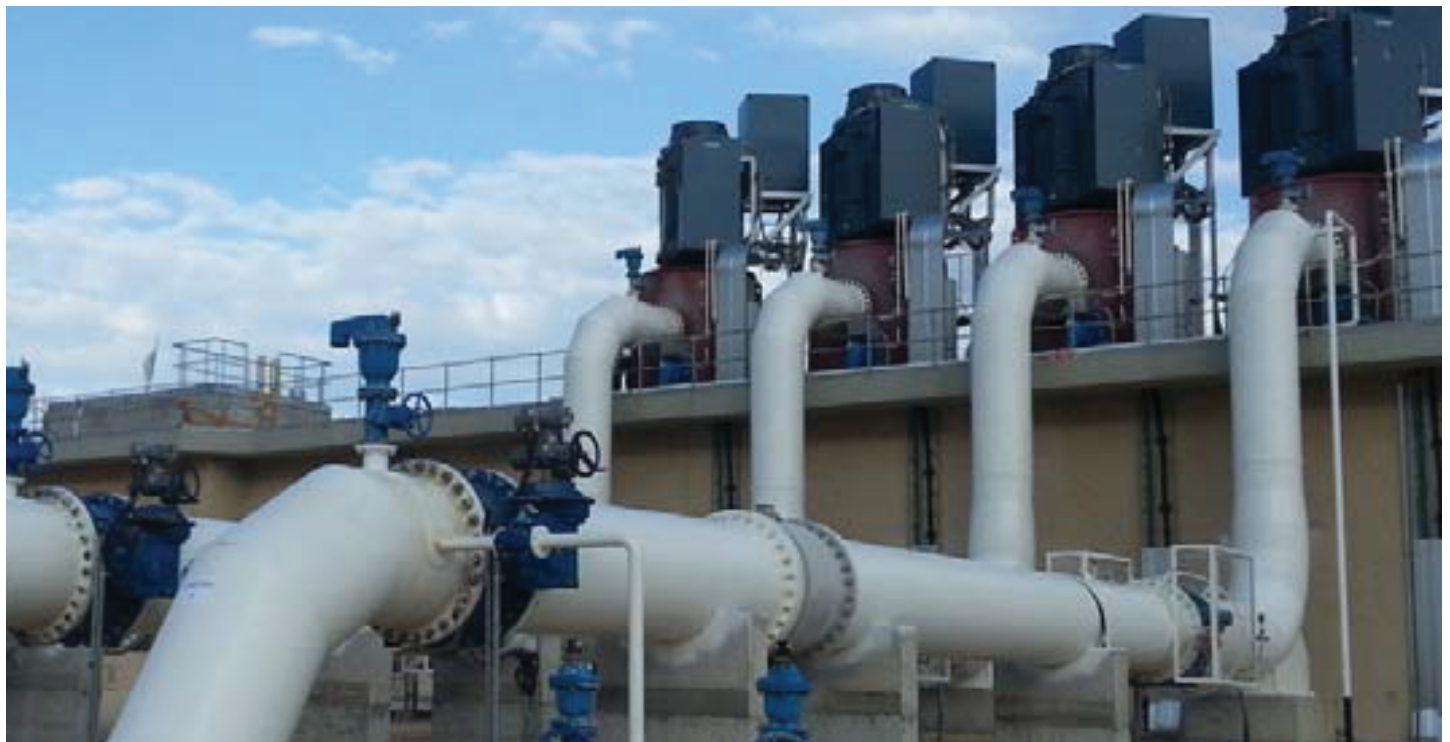
Water pump station at Mekorot Israel
