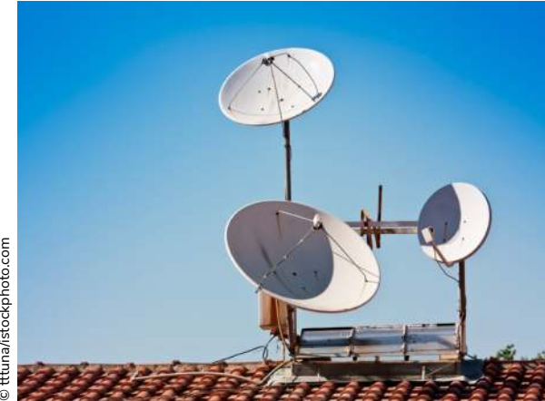
An example of SATCOM fixed antennas installed on a house roof
