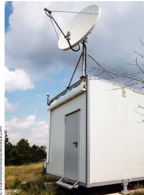
Satellite antenna of small observation station
