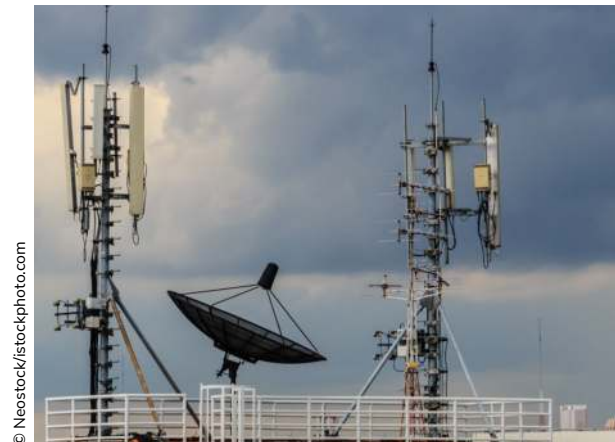
SATCOM backhauling supporting a terrestrial network cell antenna
