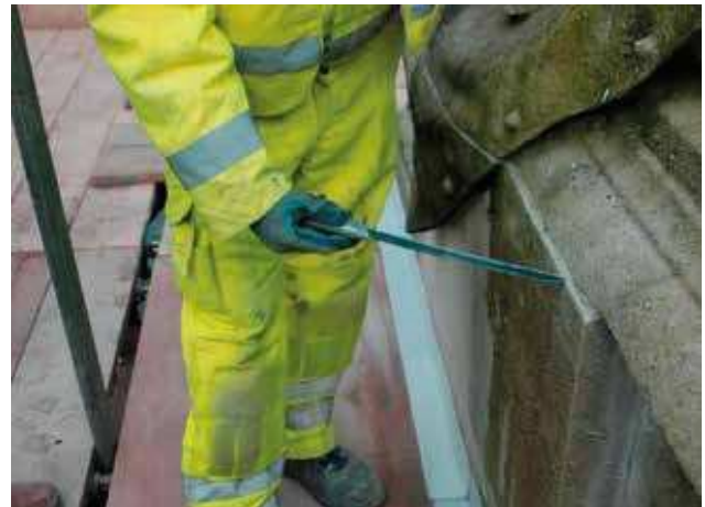
Fig 17 Removing the catafalque: cutting through the mortar joints with a tungsten carbide grit edged saw
