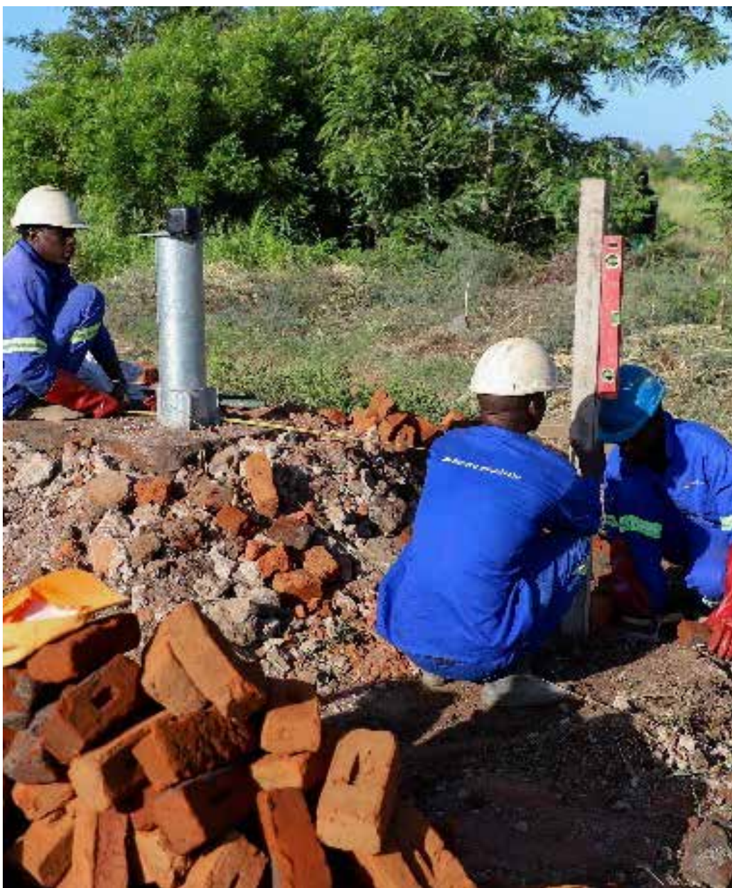
■ Figure 8: Casing around the pump high enough above the maximum floodwater level
