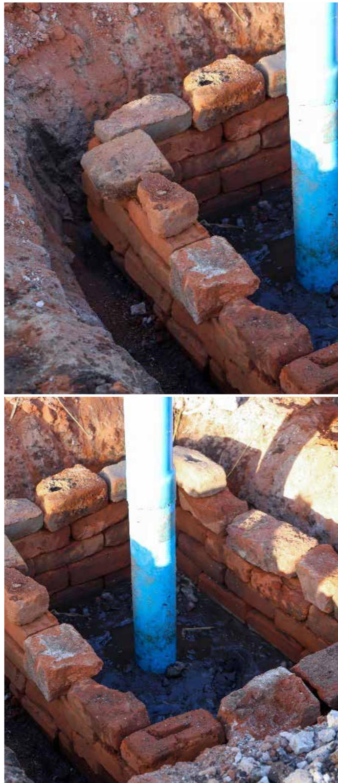
Figure 7: Protective cap of PVC lining over the pump cylinder extending below the surface to create a barrier against floodwaters.
