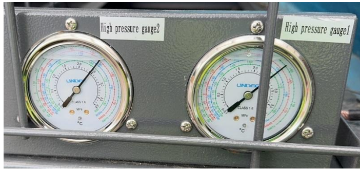
Picture 2 - Compressor Gauges
