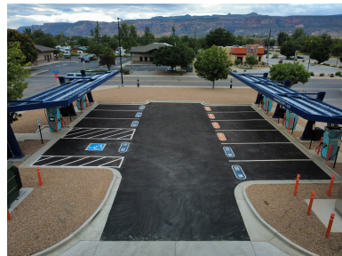
EV charging plaza. Fresh asphalt, custom EV stencils, ADA-accessible charging bays.
