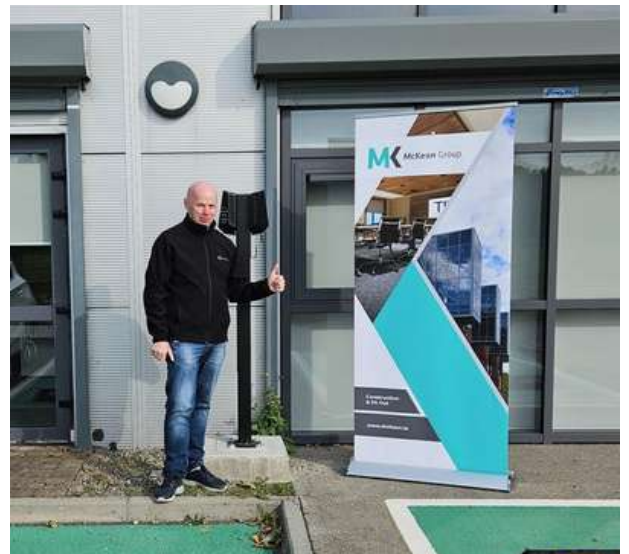
EV Chargers Installed at HQ
