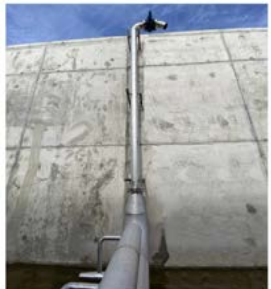
Backflush Header and Valve
