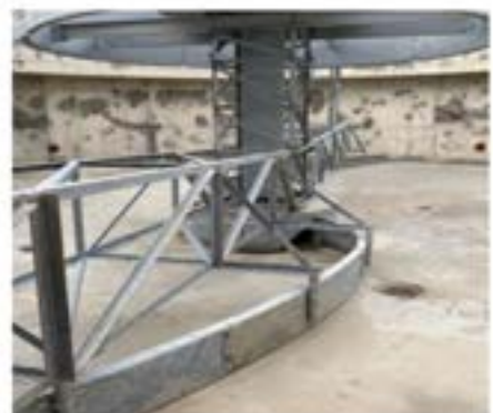
Spiral Blade Clarifier
